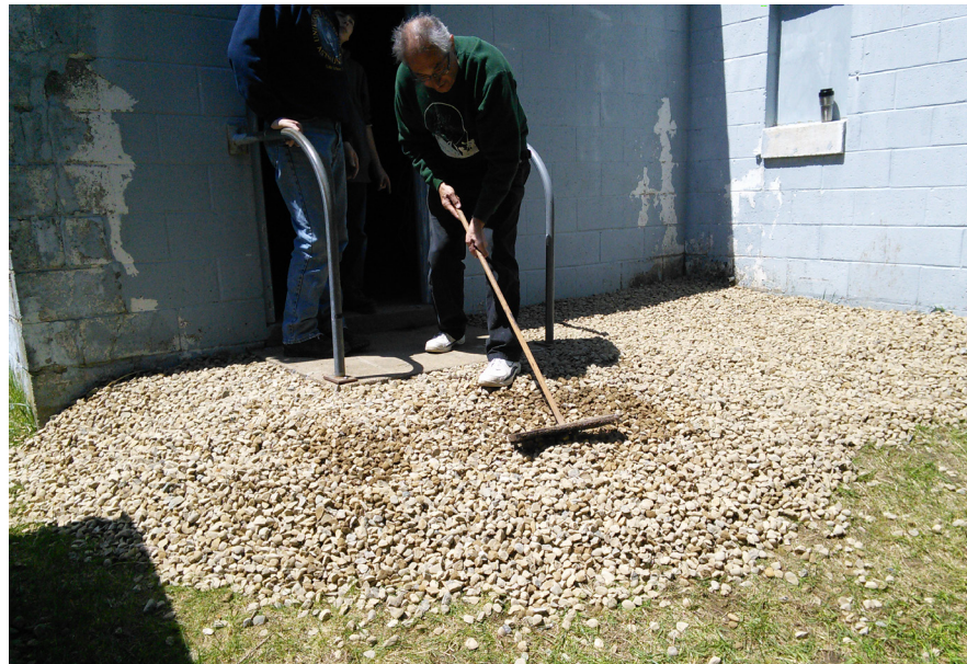
Observatory Director Jack Brisbin rakes out limestone aggregate at the Observatory's 2014 Spring Cleaning Day. The limestone ramp makes for a safer entrance to the building and the strip of it around the foundation has improved drainage.
