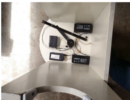
Inside of base showing batteries, azimuth encoder, encoder bluetooth box, switch box, and encoder reference bars.
