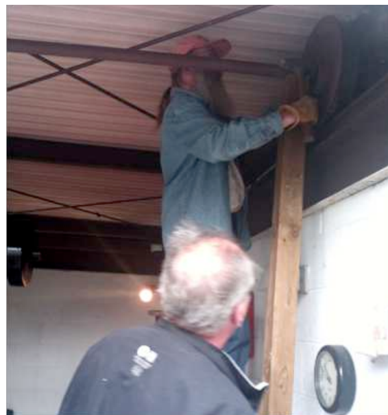
Kurt Hillig drives a wheel of the Observatory rool-off roof into place as Observatory Director Jack Brisbin advises.
