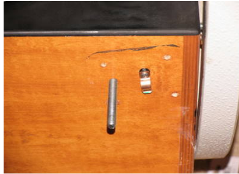
Truss Block Removed to Show Electrical Tab
